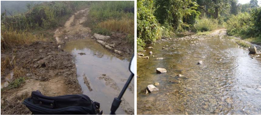
Picture 6: Road conditions to Mok Khuan (left) and Houy Hok (right) village in dry season
