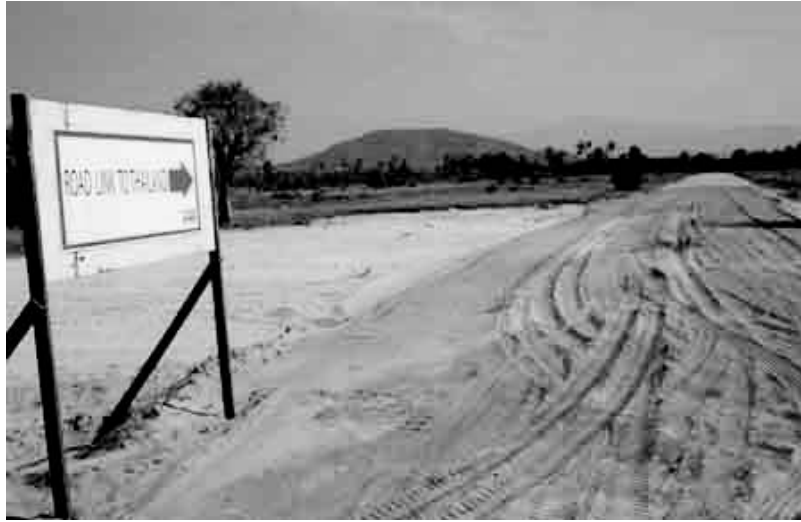
Road construction from the Nabule area to the Myanmar-Thailand border through Yebyu. Source: Taken by the author on July 20, 2010.
