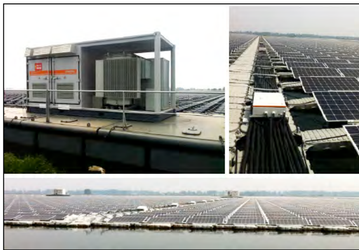
Figure 0-30. The standardized design for Sungrow floating PV system, with unit floating array block of 2.5MWac. The central inverter, switch gear and transformer are containerized and located
