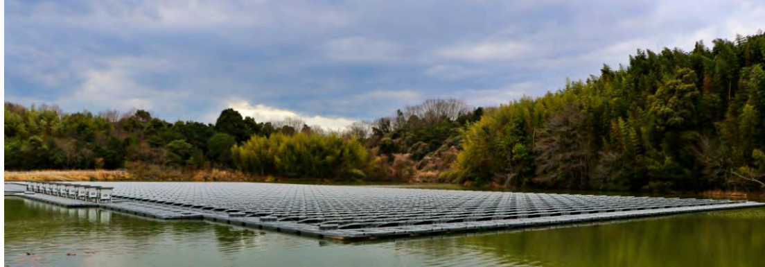
Figure 0-32. Floating Smart PV Plant, Kasai-shi, Hyōgo, Japan, where string inverters are mounted directly on the floating platform.
