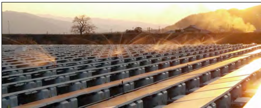
Figure 0-13. Floating PV system with active cooling, which may further enhance system performance and energy production (demonstration system built in Japan by Ciel et Terre).
