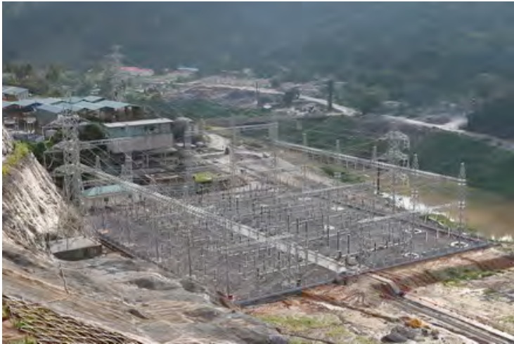
Figure 0-3. Xe Kaman 1: switch yard with transmission.
