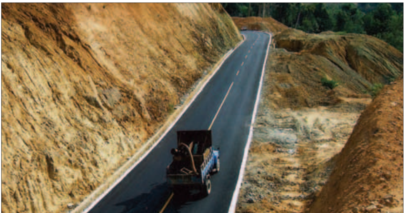
Chinese road builders returning to China along the Myitkyina to Tengchong highway; May 2007
