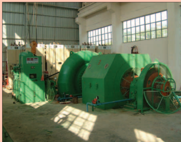
Mali hydroelectric plant
