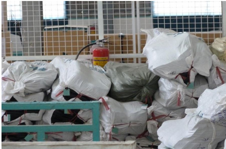
© Photo by DoLVT/MDG-F: Pile of products and materials block the access way to the fire extinguisher
