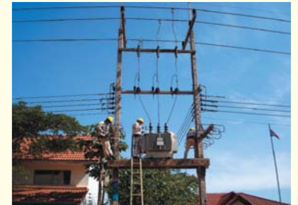
Osmach Electricity Line
