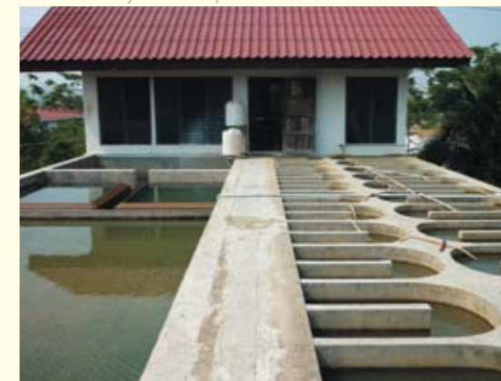
Osmach Water Treatment Plant
